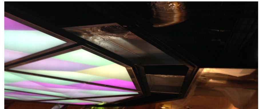
Casino exhaust duct work
