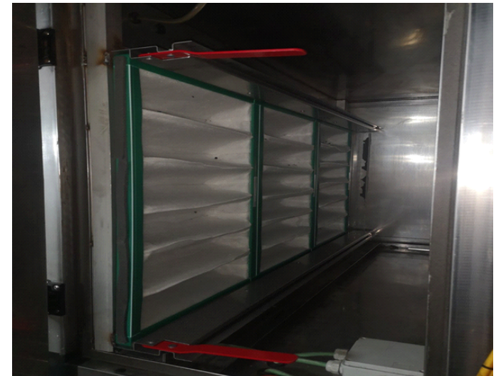
Manufactured frames for air filters
