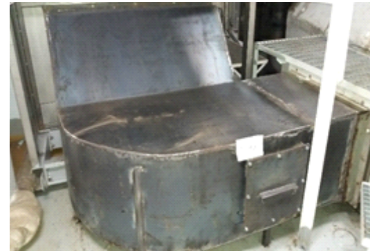
On site manufactured duct
